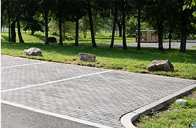
Four Mile Run incorporates permeable pavement, a form of green infrastructure, in a parking lot to reduce runoff from heavy rain. Permeable pavement can also help filter out pollutants that contribute to water pollution. (City of Alexandria)
