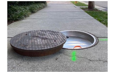
It's a change that likely won't go noticed by many Alexandrians, but the city is making an adjustment to its manholes that could have an impact on flooding during storms.
