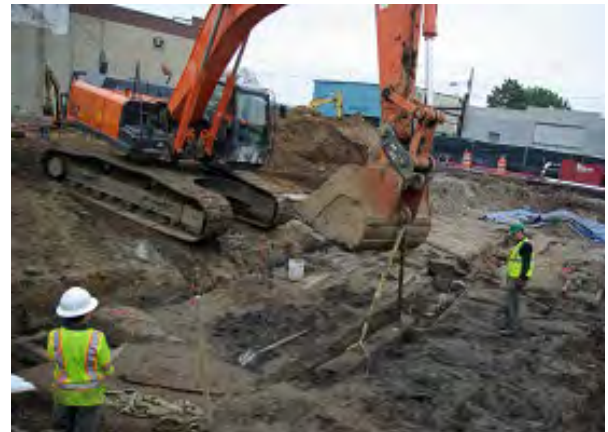
Above right: Lifting the summer beam with the help of the backhoe.
