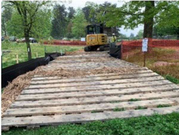
Tree mats used for equipment access at the Fort Ward picnic shelter pathway
