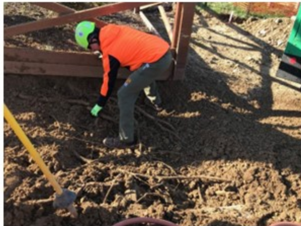
Air spading loosens compacted soil, exposes tree roots, and keeps critical root systems intact. This application was used for sidewalk construction at Ewald Park
